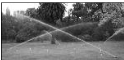
Right: Early auditing program of sprinkler system using recycled pet food tins as catch cans
